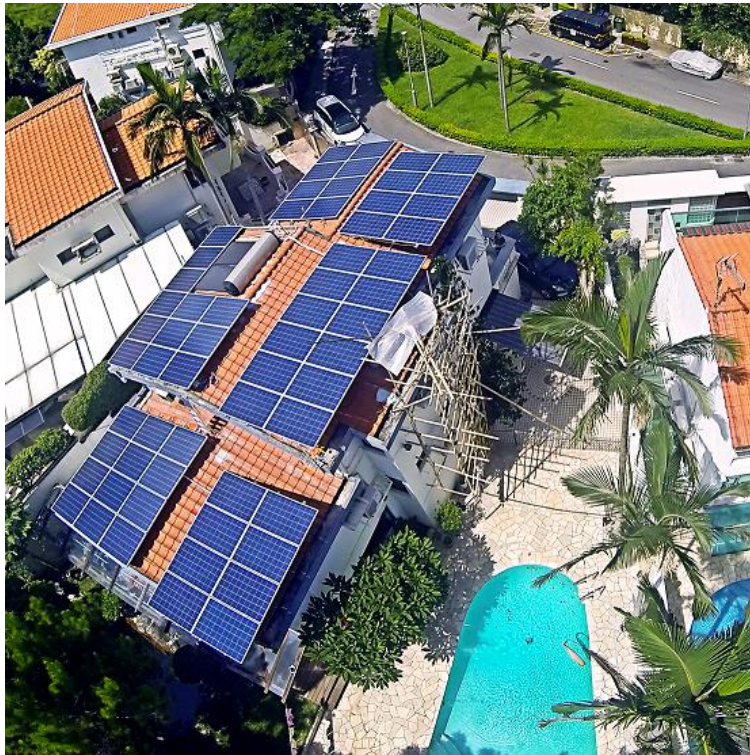
Hon Lok Yuen 15kW On-Grid System
