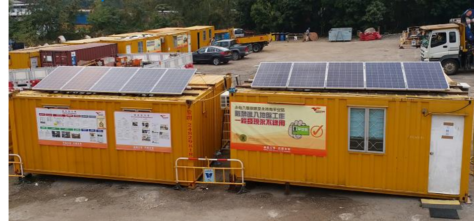
Sheung Shui 2.5kW On-Grid System
