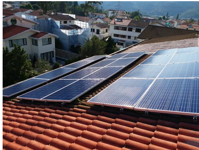
Hon Lok Yuen 5kW On-Grid System
