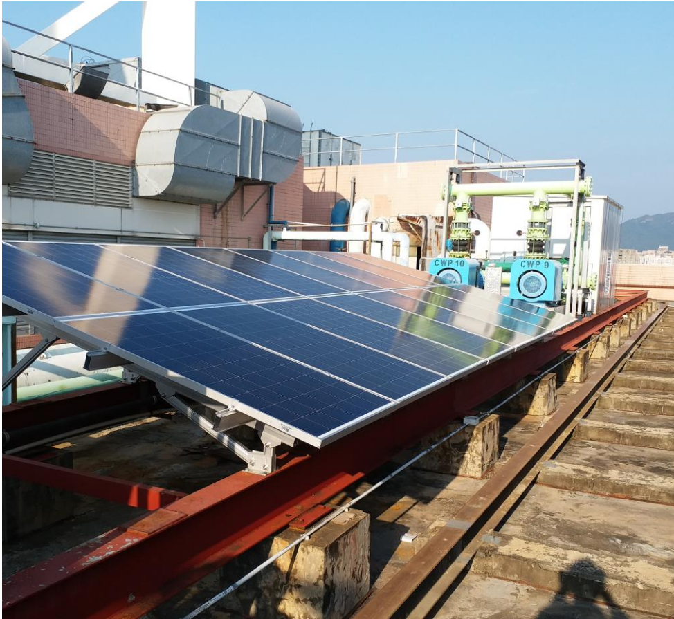
Sheung Shui Commercial Building 9kW On Grid System
