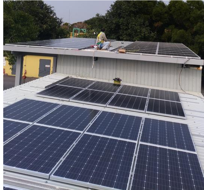
Government Project 30kW On Grid System
