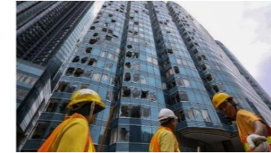
Damage in Whampoa
