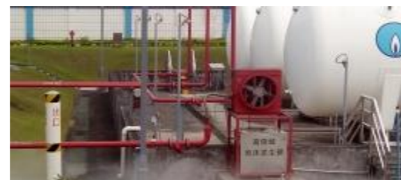
Confirm Pump Capacity
