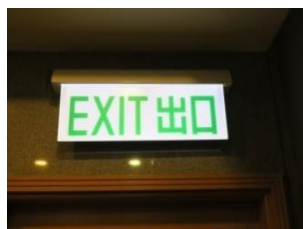
LED "Exit" sign
