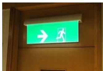
LED "Exit" sign
